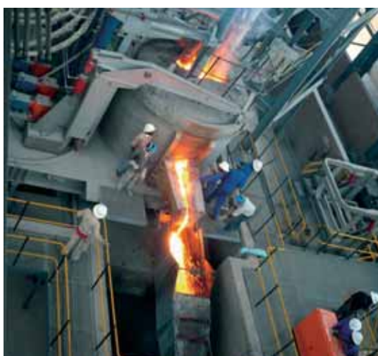
MVA AC ARC Furnace, DRC
